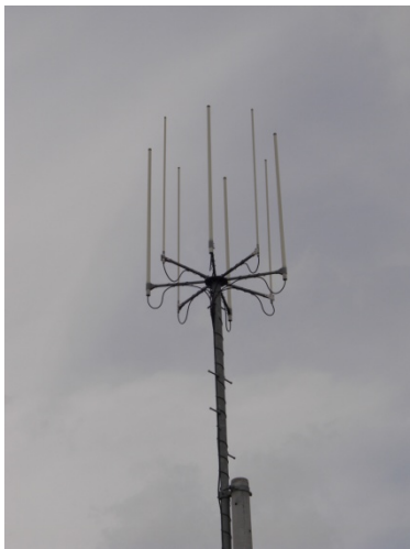
A Smart Antenna used at a PHS base station
